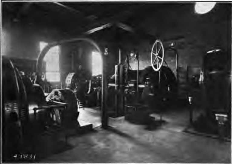
MORRIS MINE POWER HOUSE. 400 H. P. WESTINGHOUSE INDUCTION MOTOR DRIVING CAGE HOIST. 400 H. P. GENERAL ELECTRIC MOTOR ON SKIP HOIST. ALLIS CHALMERS SYNCHRONOUS MOTOR DRIVING AIR COMPRESSOR.
